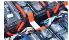
Connection resistance of battery busbars
